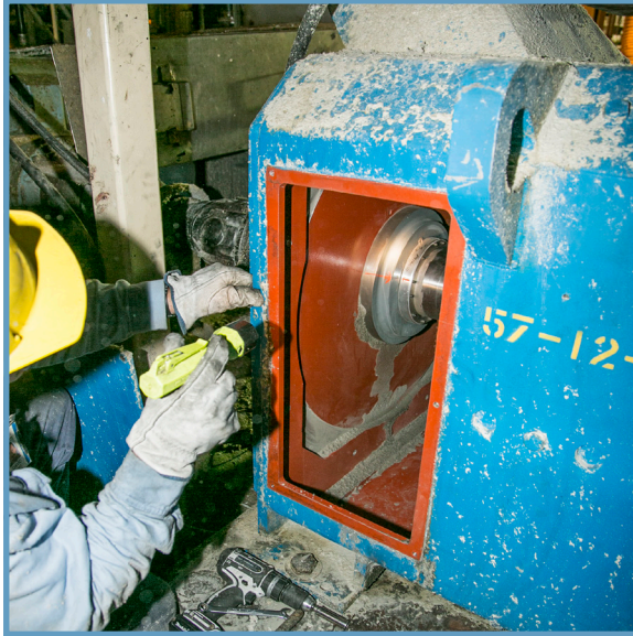
Inspecting the recently installed AEGIS® PRO Bearing Protection Ring on a key motor at the Midwest paper mill. Designed to close around the motor shaft, the split-ring PRO was installed without decoupling the motor.
