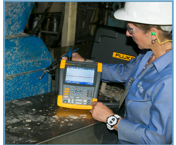
Once the AEGIS® PRO Bearing Protection Ring had been installed and the motor restarted, an AEGIS® technician confirmed that motor shaft voltages were minimal using an oscilloscope. A special "pigtail" lead allows maintenance personnel to periodically check the voltages (and therefore the likely condition of the bearings) safely and easily, without exposing the shaft. The ring has been diverting potentially damaging voltages to ground since it was installed.
